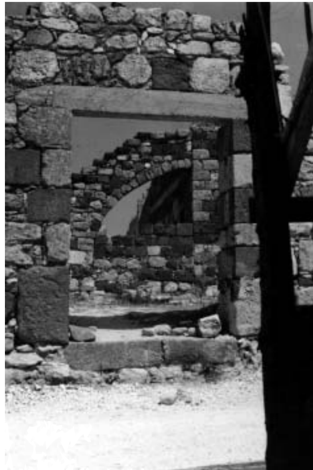
FIGURE 6. Effects of gentrification at Umm Qais: vacant and deteriorated courtyard houses and sterile but picturesque environments.
